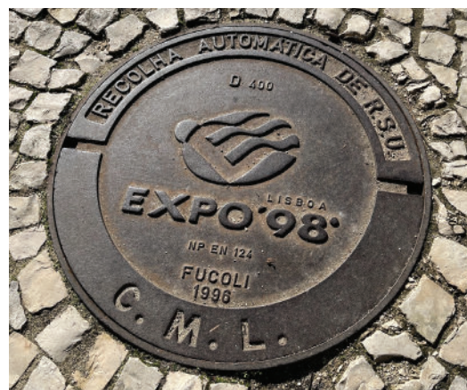
One of the underground access for pipes in the area (used for O&M)
