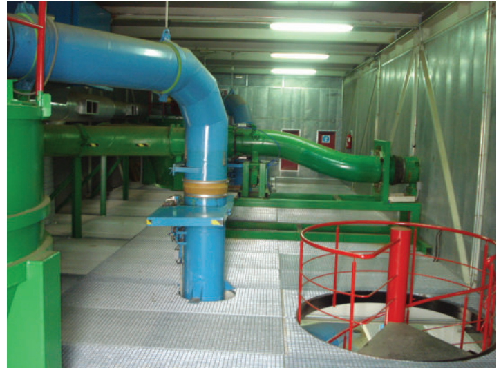
Inside of the Envac waste collection terminal
